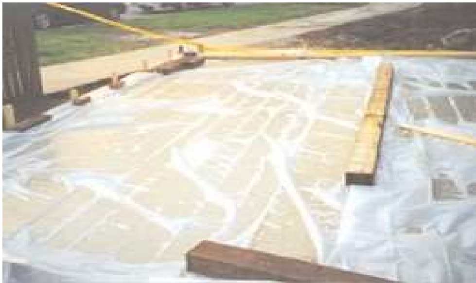
Figure 6: Polyethylene film is an effective moisture barrier for curing concrete and easily applied to complex as well as simple shapes.
