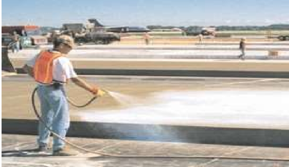
Figure 7: Liquid membrane-forming curing compounds should be applied with uniform and adequate coverage over the entire surface and edges for effective, extended curing of concrete.
